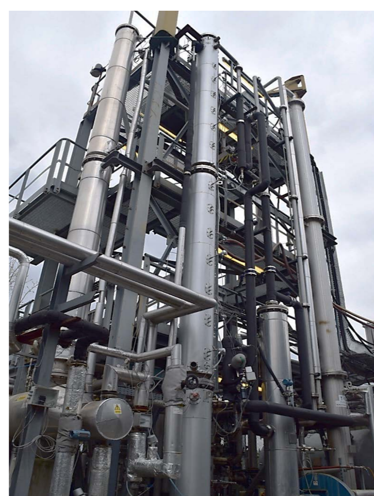
FIG 3: PACT POST-COMBUSTION CO 2 CAPTURE PLANT.
