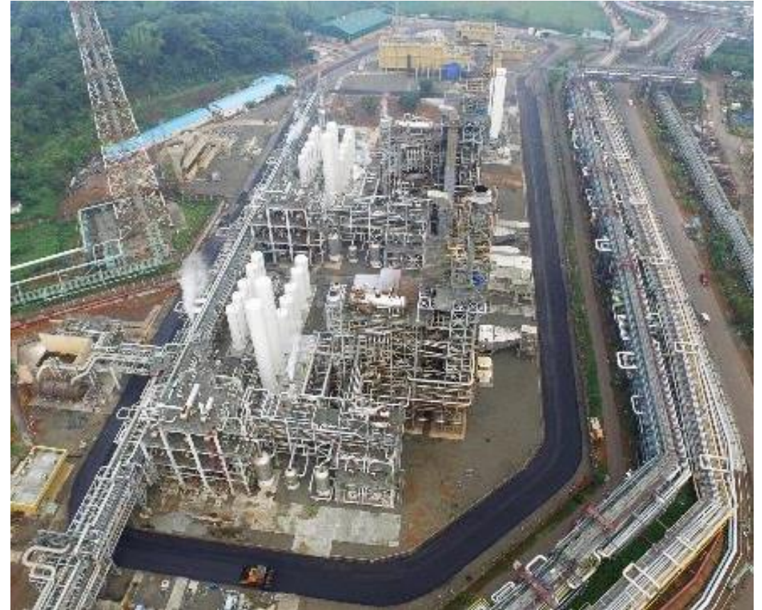
Kochi (India): First-ever twin steam methane reformers designed and built by Air Products with a combined capacity of 16.4 tons per hour of hydrogen production.
